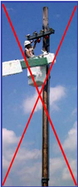
Eliminate Specialty Equipment
